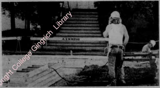
Construction workers pave a new fire lane in front of White Chapel photo by R. York
