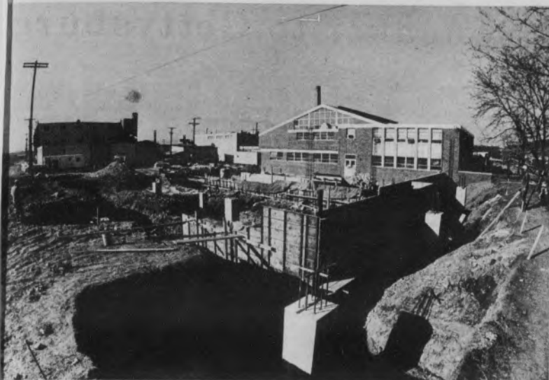
Construction continues on the new Lifesports complex adjacent to the Bollman Center. The facility is expected to be completed in 1983.
