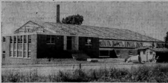
The new physical education building is pictured above as it looked this week during a construction strike which threatens to prevent completion of the structure by next September. All materials and equipment are on hand and the main floor area has been nearly completed, but unless work is resumed within two weeks, the building probably will not be finished on schedule. Current plans call for an addition to the building approximately 20 x 80 feet in size and designed to provide for small gym classes and serve as a lecture room and cloak room. (Albrightian Staff Photo.)
