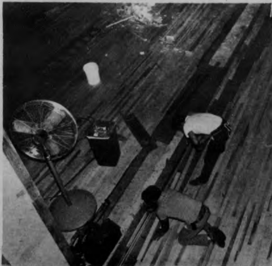
Workmen put the final touches on the fresh air circulation system in the Lifesports Center.
