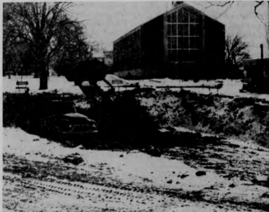
HAUL AWAY —Workmen have been busy for the past three weeks hauling away part of the campus. A steady flow of trucks carried away ground from the area where a new nearly one million dollar library and administration building is to be built. Excavation continued despite extreme cold and snow.
